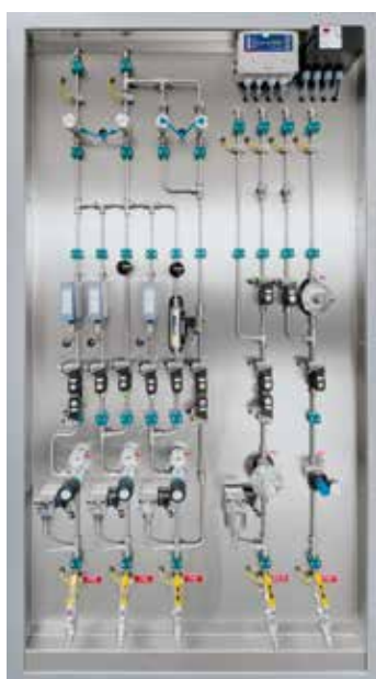
Gas management system
