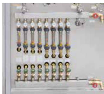
Cooling water distribution
