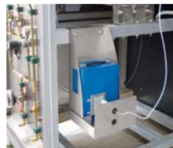
Acid pump for nitric acid
